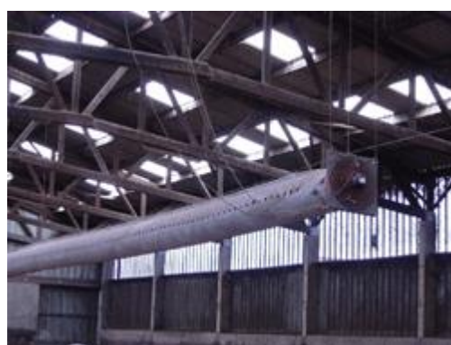
Figure M14.1. Duct for dispersing the tracer gas within a building (source: INRA)
